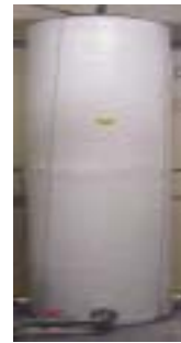
Hot Water Holding Tank
